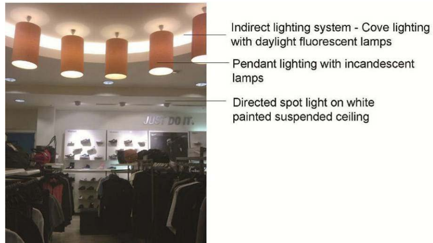
Figure 5.25: A view from the sport wearing department and its features- Coordinates on plan H13
