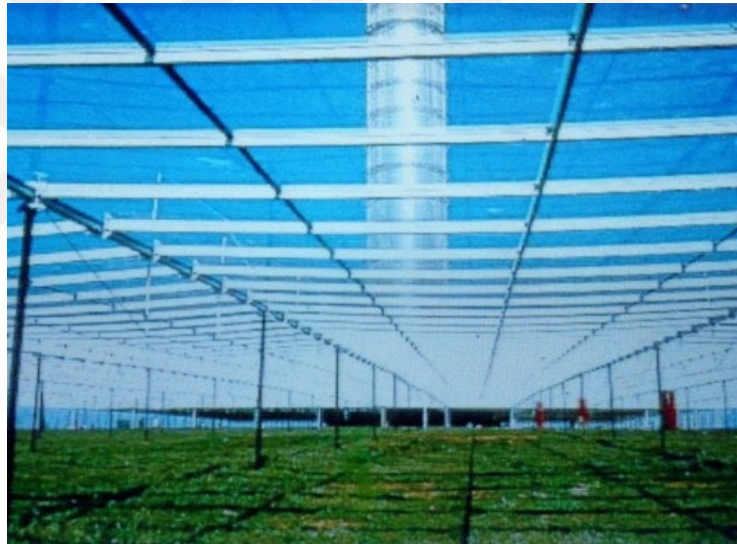
Figure 1.7: The collector structure of the Manzanares SCPP [8].
