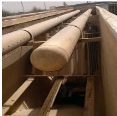
Figure 1.2 Inside sedimentation basin for compact unit
