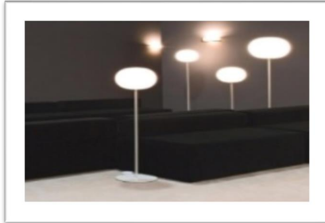
Figure 2.19: Diffused Lighting Fixtures (“Lighting”, 2012)
