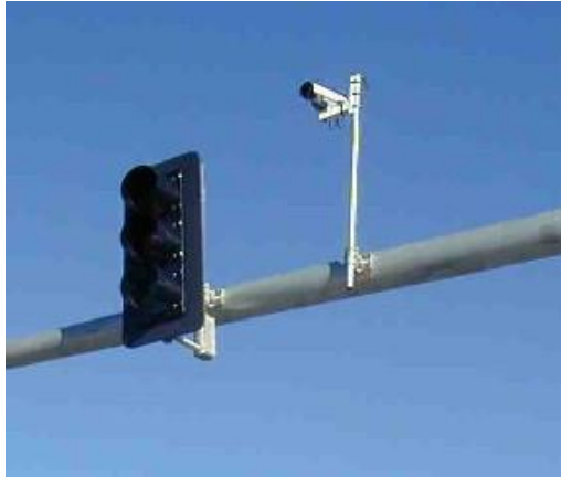
Figure 2.10: Control center cameras
