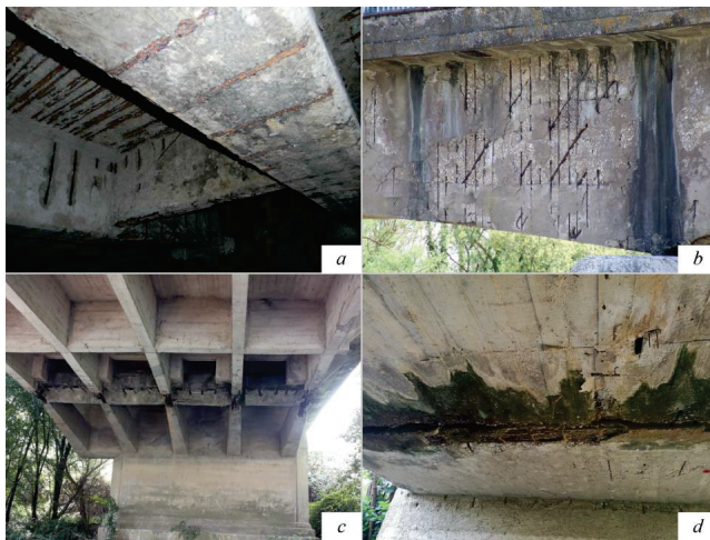
Figure 2. Deck degradation state: New Bridge in Capua (a), Bridge in Castel Morrone (b), Margherita Bridge in Dragoni (c) and Bridge in Aliano (d).
