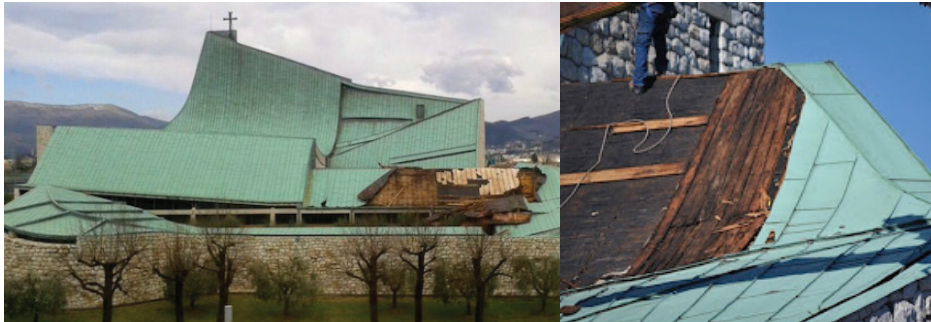
Figure 1. The San Giovanni Battista Church realized by Michelucci: the damage of the gallery of Nation roof after the storm
