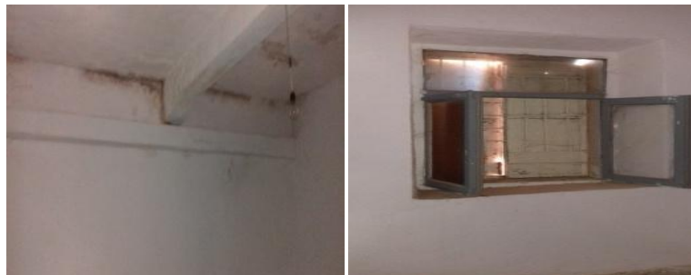
Figure 55. Shows the window and the roof from the inside without a change in the Italian style
