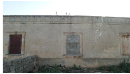
Figure 58. Showing the right side of the house and the windows cracked in the presence of the wall and not fit for habitation
