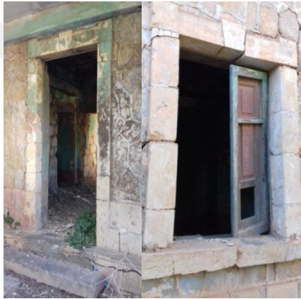
Figure 66. Show the door and window with a frame which shows the Italian style
