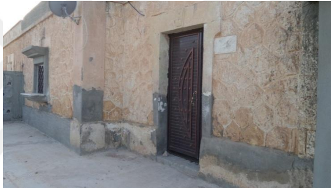
Figure 25. The front of the house shows the change only in the door
