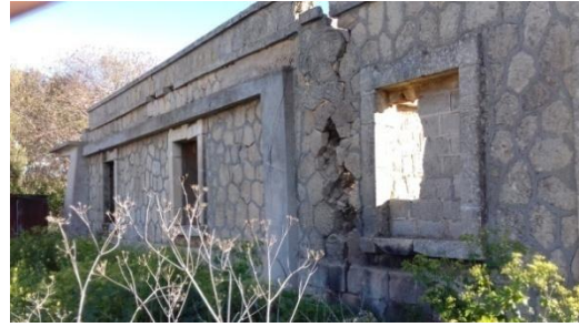
Figure 65. Showing the right side of the house with the windows also cracked the wall
