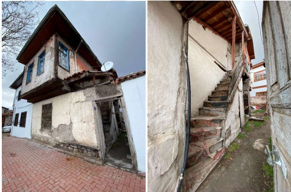
Figure 25. Hamamarkası Region, Views of the Old Building Bay Window, Court, Stairs, Wood Pole, Eaves, Gutter (Buildings In Upper Photo) (Author's Archive, 2021)
