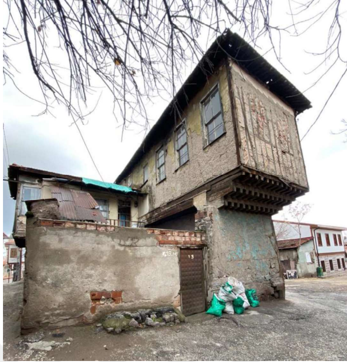
Figure 46. Ankara Hamamarkası Region, 3-Step Corbelling Bay Window (Buildings Photographed By Tuncer, Figure x.y) (Author's Archive, 2021)
