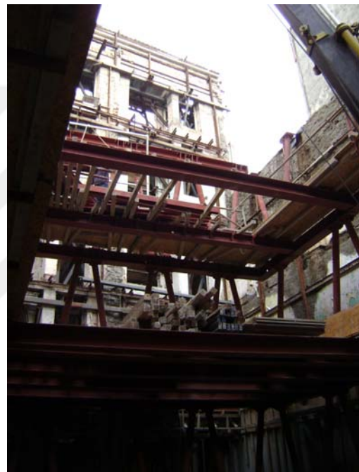
Figure 5.3 Diagonal structure is being erected as the steel beams are placed between the layers (GAD, March 2008)
