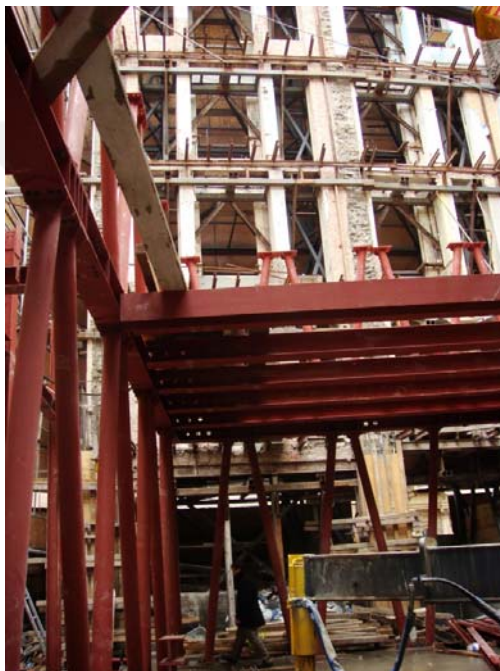
Figure 5.2 Steel supports are used to keep the frontal facade standing (GAD, February 2008)
