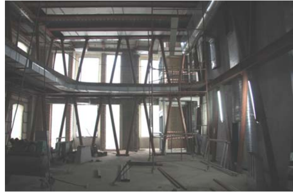
Figure 5.13 Elevator structure was installed while construction of 2 nd and 3 rd floor gallery void was still ongoing (GAD, November 2008)
