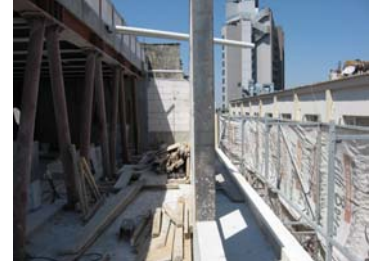
Figure 5.8 Construction of structure reached as high as the terrace level (GAD, August, 2008)
