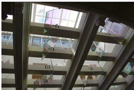
Figure 3.59 Salt Galata's mirror panels (heliostats)
