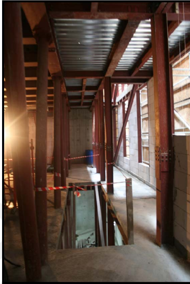
Figure 4.59 Diagonal steel structure is seen on the left side, I steel columns are seen on right side, gas concrete blocks are seen on right front, steel right profiles used in horizontal are seen at the top
