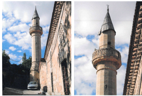
Fig. 3. Degradation, Decay and cracks occurred on the minaret.
