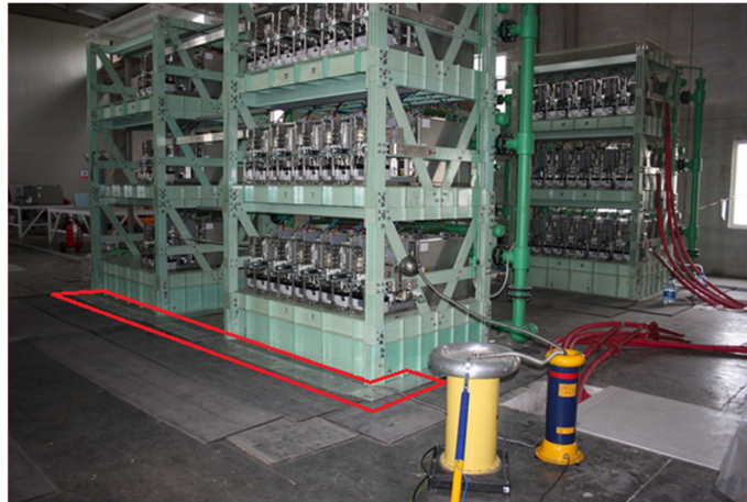
Figure 20. Grounding grid with metallic plates.
