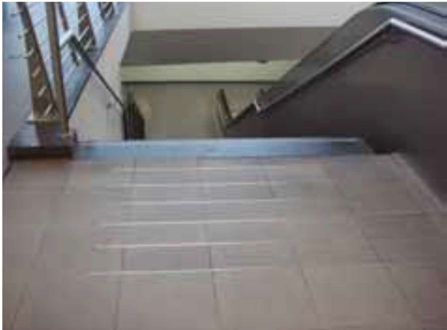
4.1.15. Embedded Metal Bars Marking the Top of a Stairway (Brussels, Belgium)
