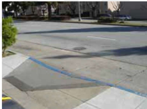
4.2.1. Shallow Grooves Cut into the Pavement before a Crosswalk (San Francisco, USA)
