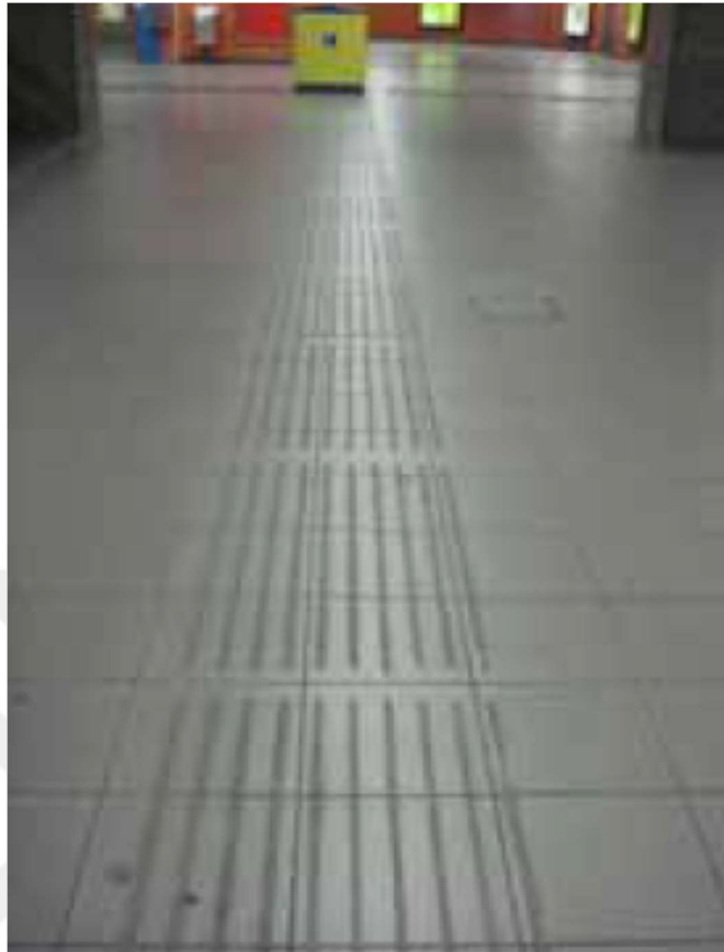
4.1.16. Embedded Directional Metal Bars (Brussels, Belgium)
